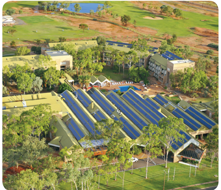
Crowne Plaza Alice Springs 305 kW photovoltaic installation (image courtesy of Crowne Plaza)
