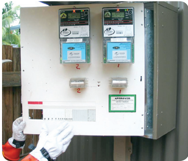
Smart meter being installed in Townsville Solar City household (image courtesy of Townsville: Queensland Solar City).
